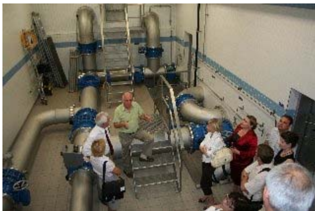
July 2008. Study tour to Switzerland. Community Water Supply in St. Gallen
